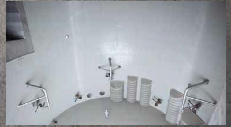
Above picture: Internal view of sump area in a flue gas scrubber built using concrete and BEKAPLAST™ including fixtures.
