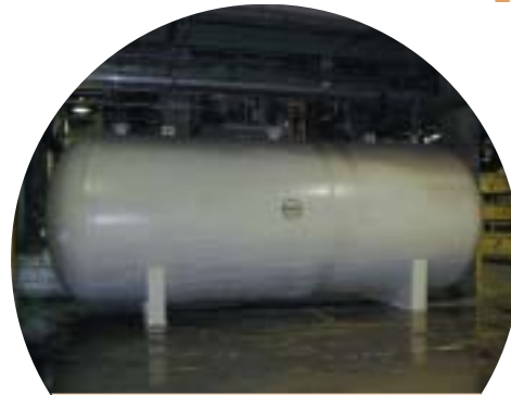
New 10,000-gallon compressed air storage tank
