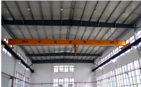
单梁桥式起重机/Single cranes
