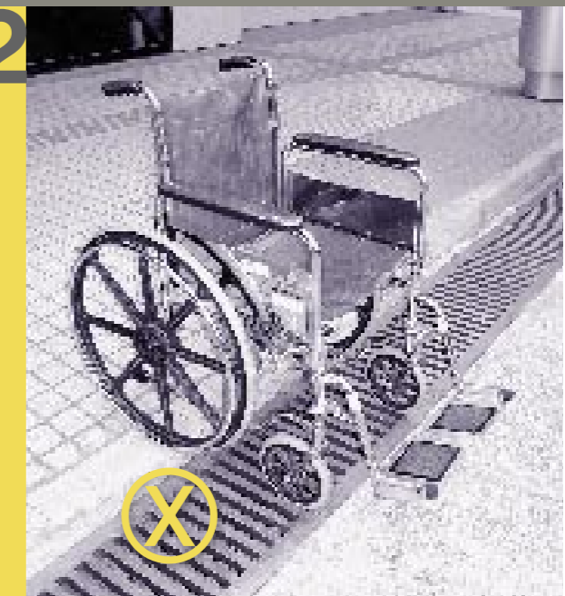
The openings for the gratings are not small enough and are also in the direction of major traffic 渠道格柵開過大且與主要行走方向平行
