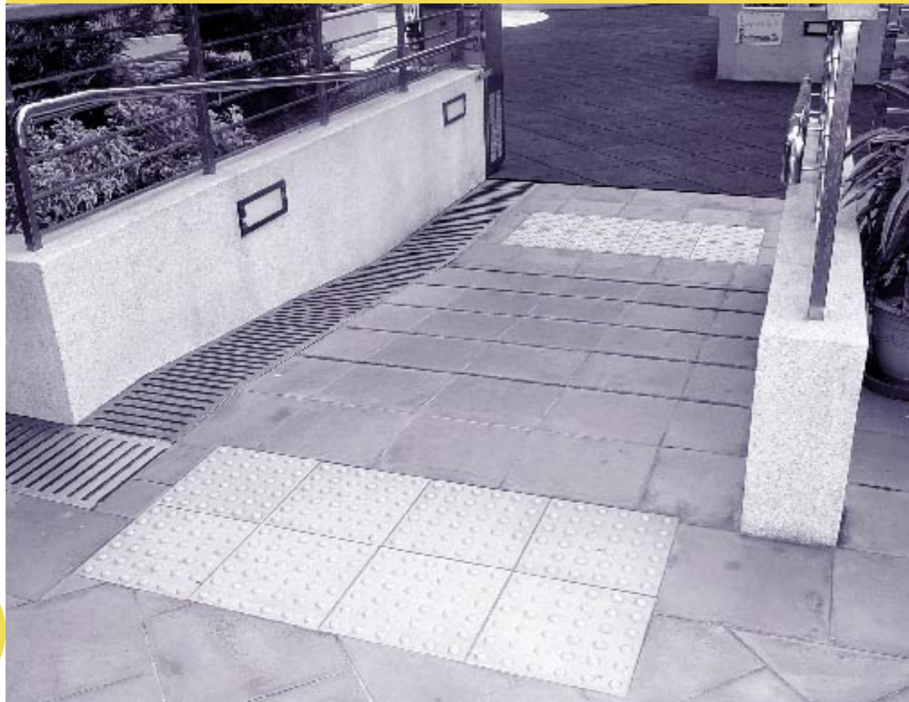
Hazard warning tiles for ramps 斜道的危險警告引路磚
