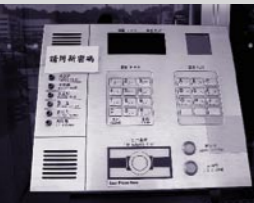
Intercom panel at building entrance 入口處的對講機
