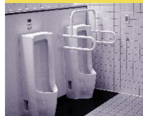
Vertical handrails for a urinal 尿廁的垂直式扶手
