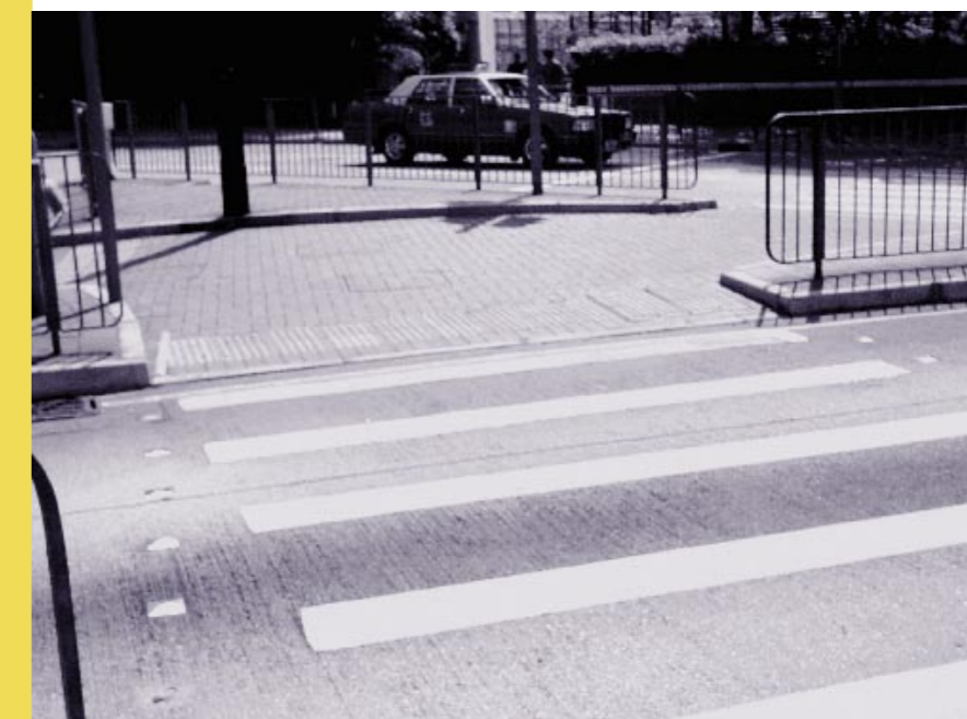
A dropped kerb with hazard warning tactile surface 有凹凸警告條紋的下斜路緣
