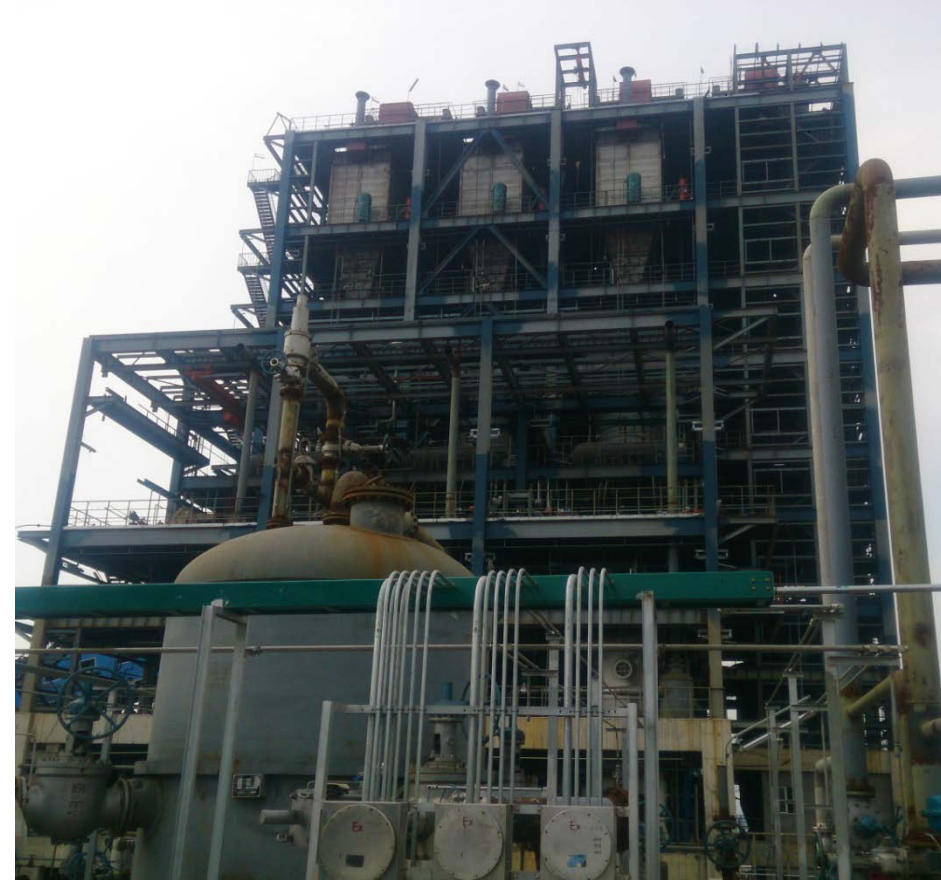
HT-L Gasifier Device ( 750 TPD )
